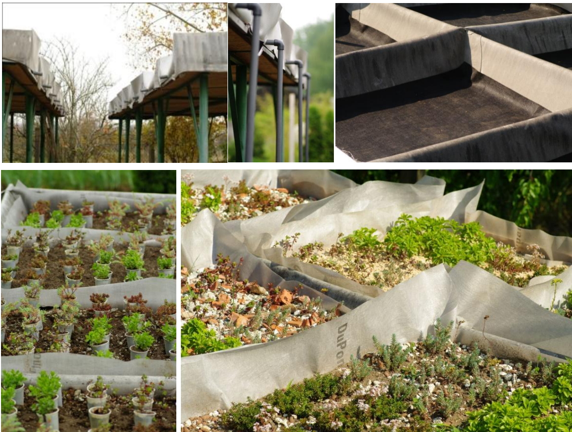
Figure 1. The two experimental roofs (a) Drainage pipes (b) Parcels with PVC insulations (c) Before planting (d) After planting (e) (Nyíregyháza, Ilona tanya)
